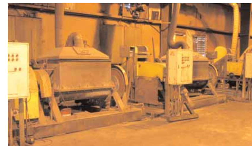
(3) Hot Mix Mixers with Twin Horizontal Kneaders
