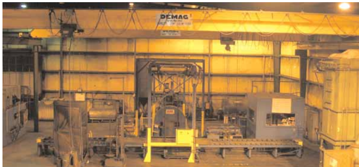
Overview of Isostatic Press Line and Demag Bridge Cranes
