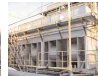
BAC 300-Ton Evap. Cond.
