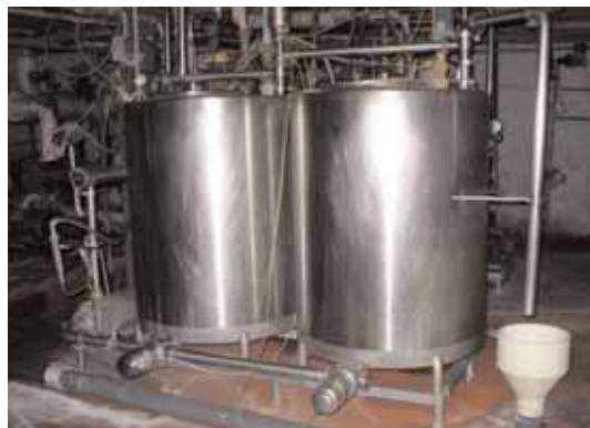
(2) 2-Tank CIP Systems
