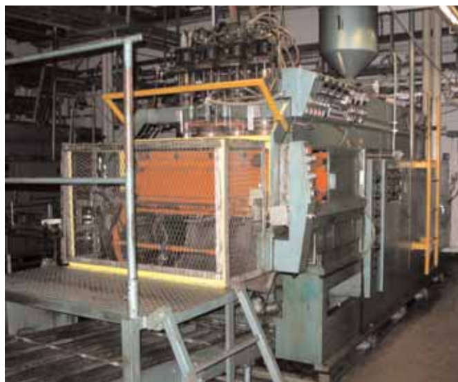
(4) Uniloy 4-Wide Half-Gallon Blow Molders
