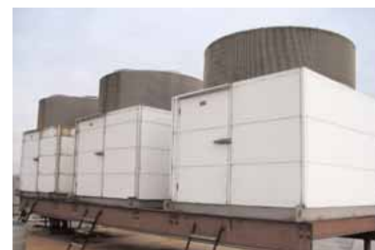
(3) Edwards Package Chillers
