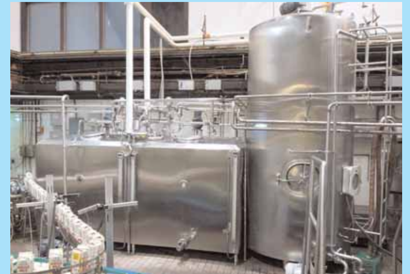
(2) Cherry Burrell 1,000 Gal. Blend Tanks Cherry Burrell 2,000 Gal. Freon Refrigerated Blend Tank/Silo
