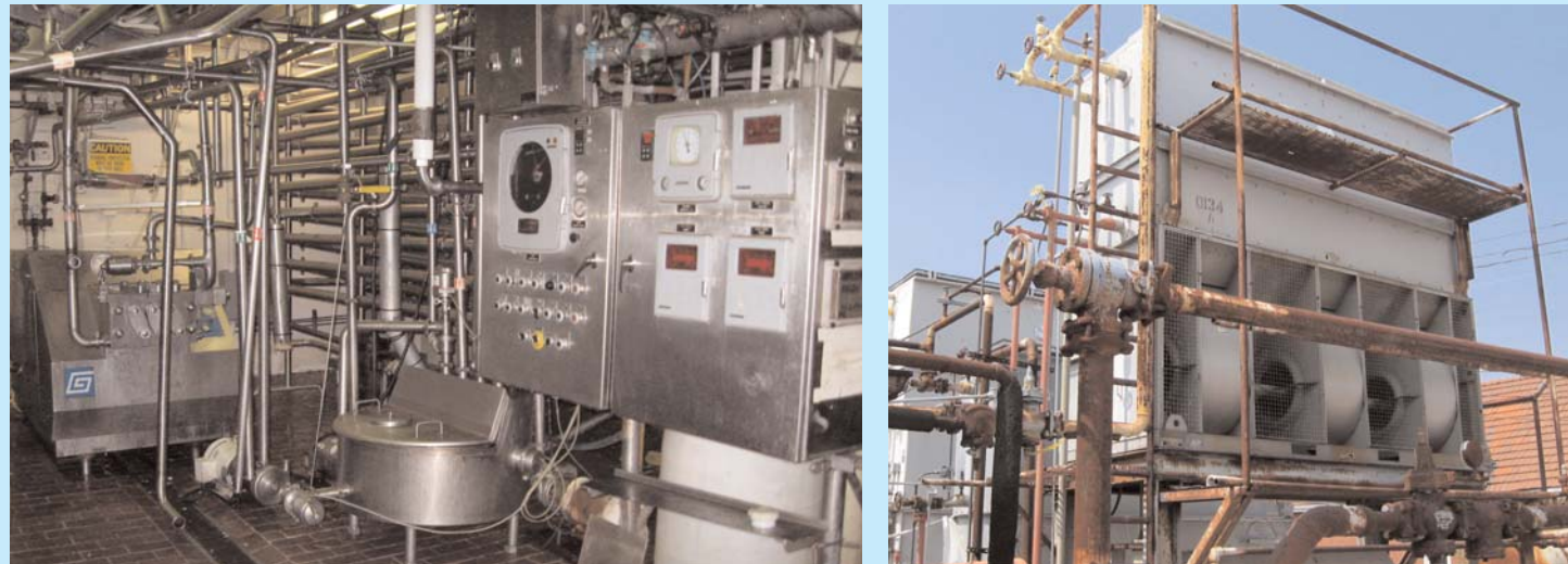
APV 4,000 gph Mix HTST System & Gaulin MS18 Homogenizer - (3) BAC Evaporative Condensers
