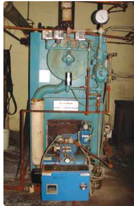
Cleaver Brooks Boiler
