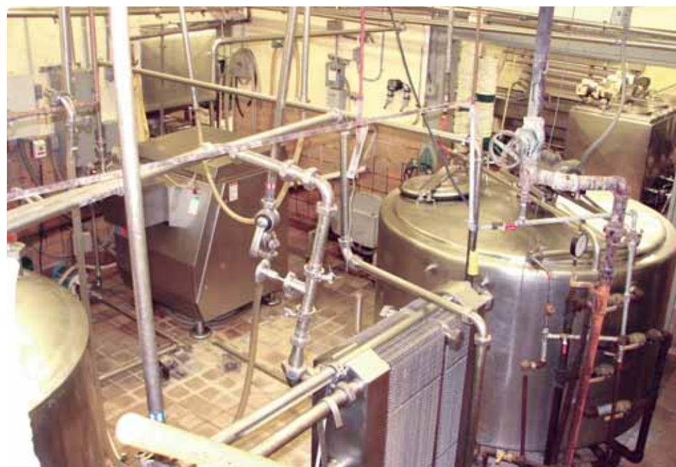
Overview of Mix System and Batch Room
