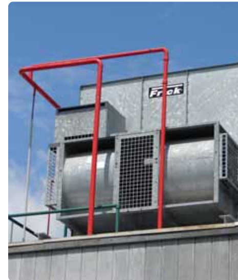
Frick Evaporative Compressor
