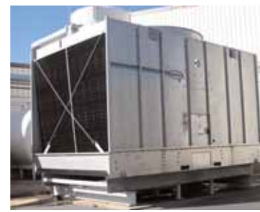
(9) Marley & other Cooling Towers
