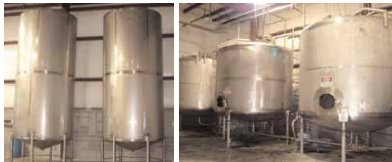
(2) 2000 Feldmeier 6k Gal. S/S Tanks - (3) 8k Gal. Sugar Tanks
