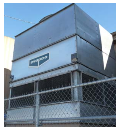
Evapco ATC180 Condenser
