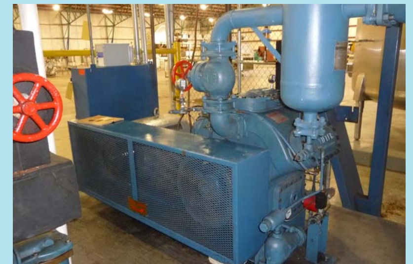
(2) Vilter 75 hp 6-Cylinder VMC440 Ammonia Compressors
