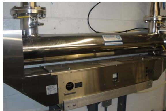
Water Treatment including Aquafine UV Light
