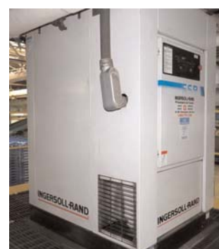
I.R. 75hp & 50hp Air Compressors
