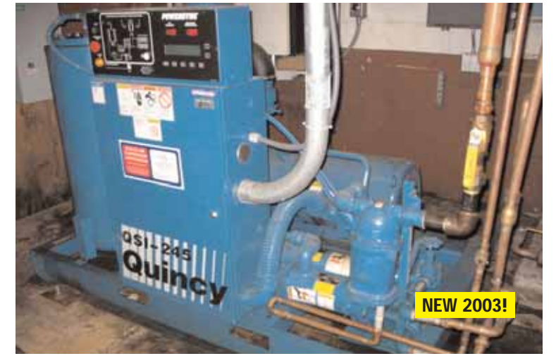
2003 Quincy 60 hp Screw Air Compressor
