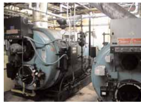
(2) Cleaver Brooks 175 hp & 70 hp Boilers
