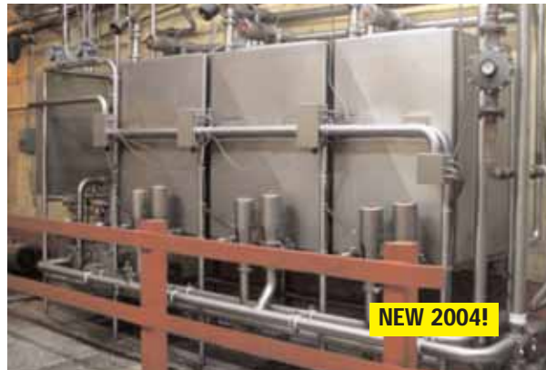
2004 EcoLab Skid Mounted CIP System
