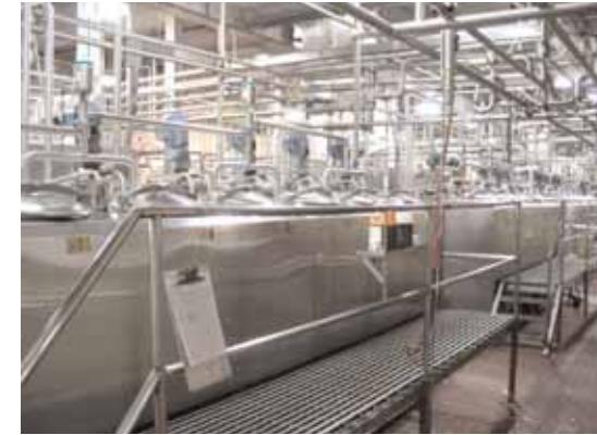
(5) 6-Compartment @ 300 Gal. S/S Flavor Tanks
