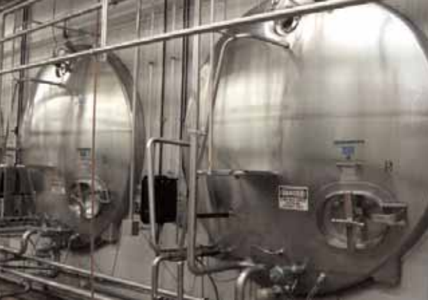
(5) Walker 10,000 Gal. Refrigerated Silos
