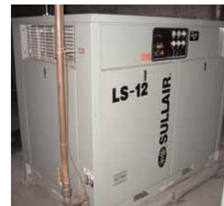
(2) Sullair Screw Air Compressors
