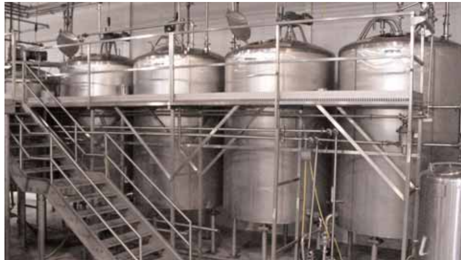
(4) Mueller 1,864 Gal. S/S Dome-Top Processors
