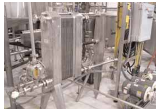
(3) APV Presses & Centrifugal Pumps
