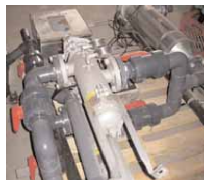
Trojan UV Water System
