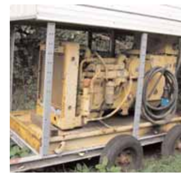
Portable Generator w/Cat Diesel
