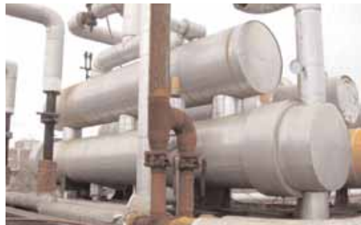
(4) Vilter, El Nickell and RVS, Shell and Tube Glycol Chillers
