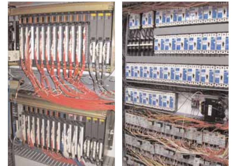
Allen-Bradley and Cuttler Hammer Controls & Breakers
