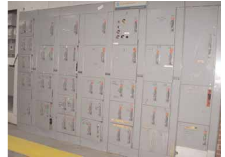
Siemens, Square D & Allen-Bradley Switch Gear
