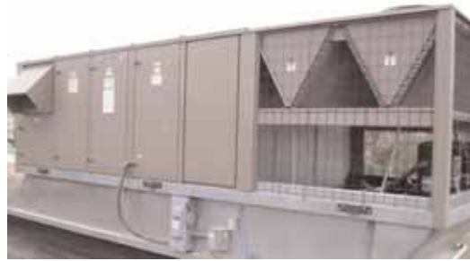
York Air Handling and Air Conditioning Units
