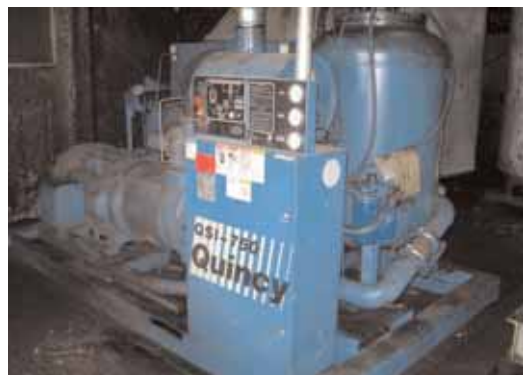
Quincy 150 hp & Sullair 125 hp Screw Air Compressors
