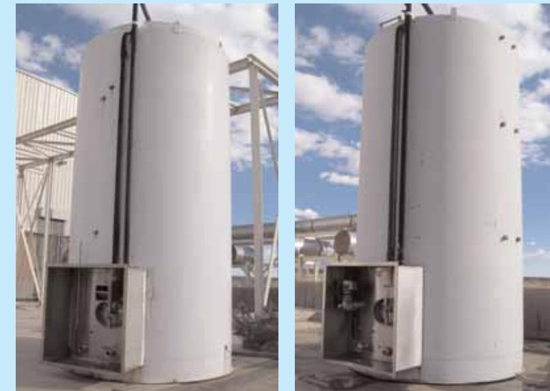
(2) Mueller 10,000 Gal. S/S Silos
