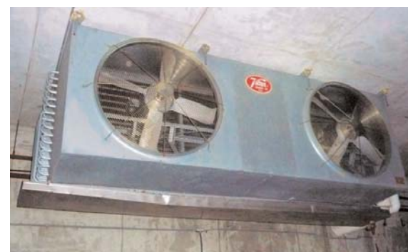
(2) Vilter & (5) Krack Ammonia Blowers
