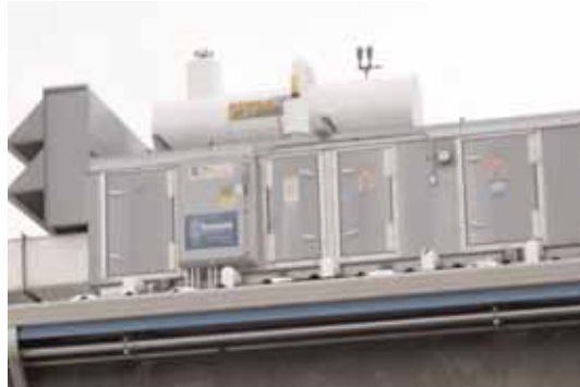
1999 King Air Handler
