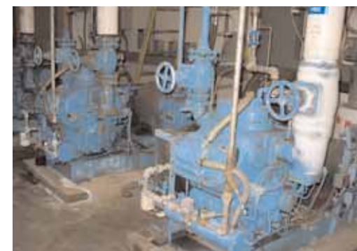
(7) Mycom 8, 6, & 4-Cylinder Ammonia Comprsr.
