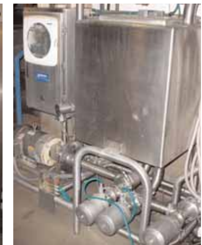
2000 AGC Cream Press HTST Controls (2) Klenzade CIP Systems
