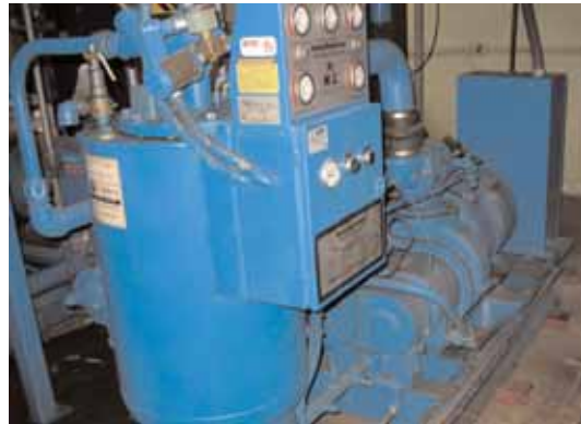
(2) Quincy Screw Air Compressors
