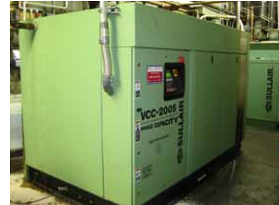
2007 & 2003 Sullair 150 hp Screw Air Compressors
