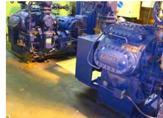
(2) 150 hp Vilter Ammonia Compressors Rebuilt 2007 & 2006! Details page 3
