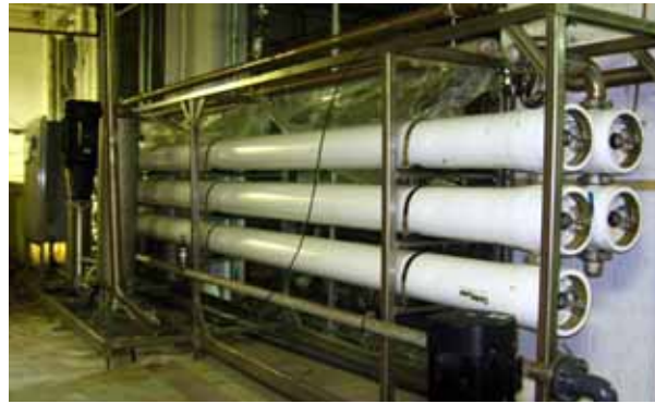
2007 Daico 100 gpm Reverse Osmosis System
