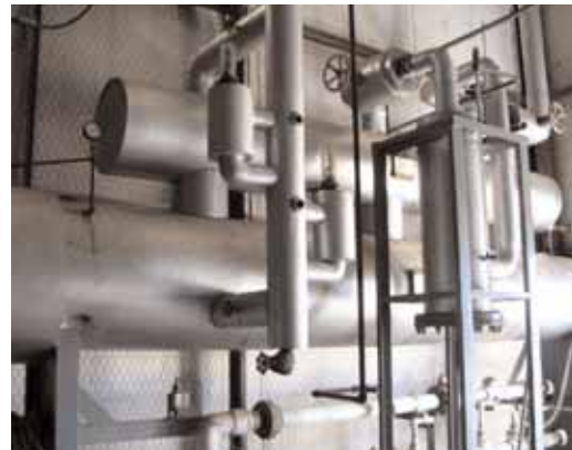
Glycol System and other Refrigeration Components
