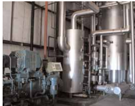
Ammonia Receiver, Ammonia Accumulator
