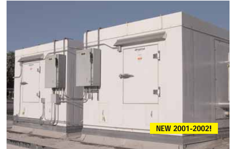
(4) 2001 & 2002 York Frigid Coil Freezer Evaporators
