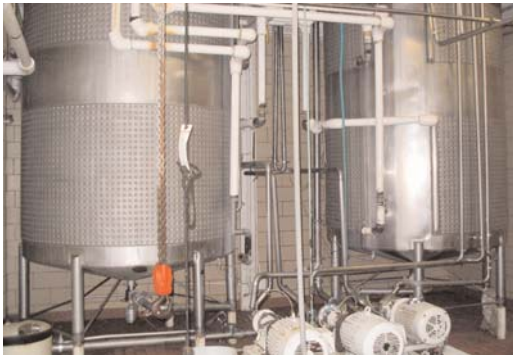
(14) S/S SILOS & TANKS
