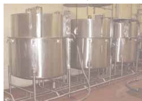
(3) Perma San 500 Gal. S/S Tanks
