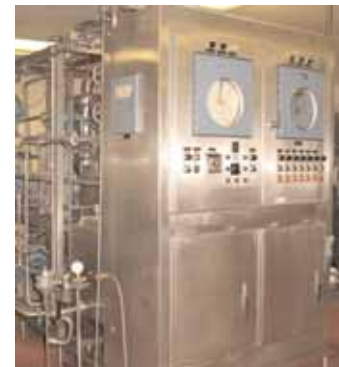
APV HTST/UHT Pilot Plant
