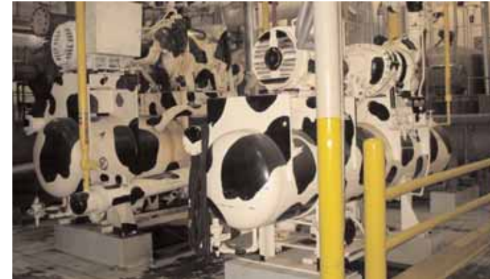
(6) FES Screw Booster Ammonia Compressors
