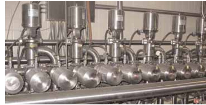
S/S Air Valves, Pumps & Pipe
