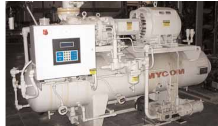
Mycom 125 hp Freon Screw Compressor
