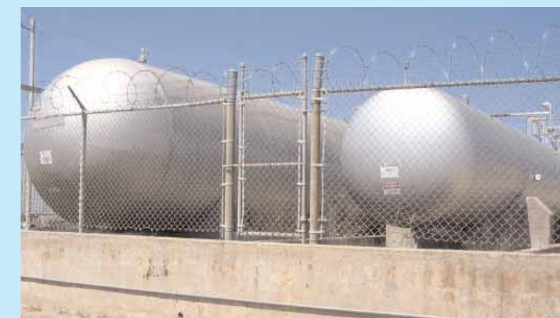
(2) 86" O.D. x 55' long Nitrogen Storage Tanks
